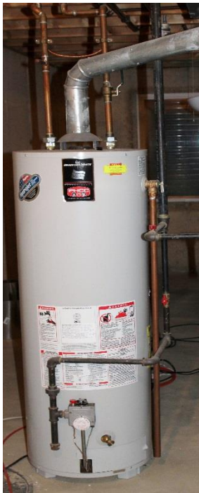
80,000 BTU/hr Water Heater
